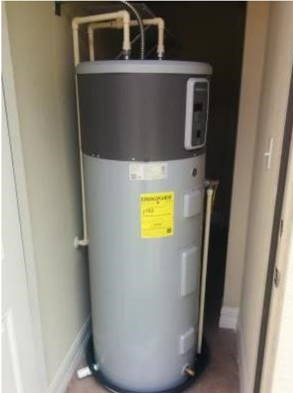
Electric Storage Tank
