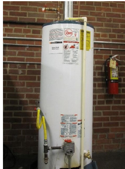
Gas Storage Tank
