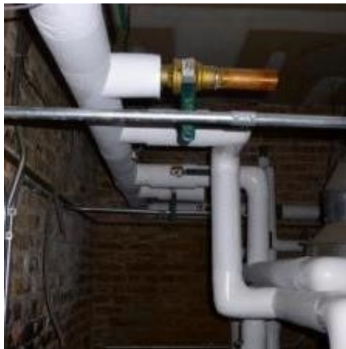
Insulate 100% of hot water pipe
