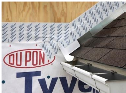
Step 5: Apply self-adhering flashing over top edge of step flashing, diverter and housewrap.
